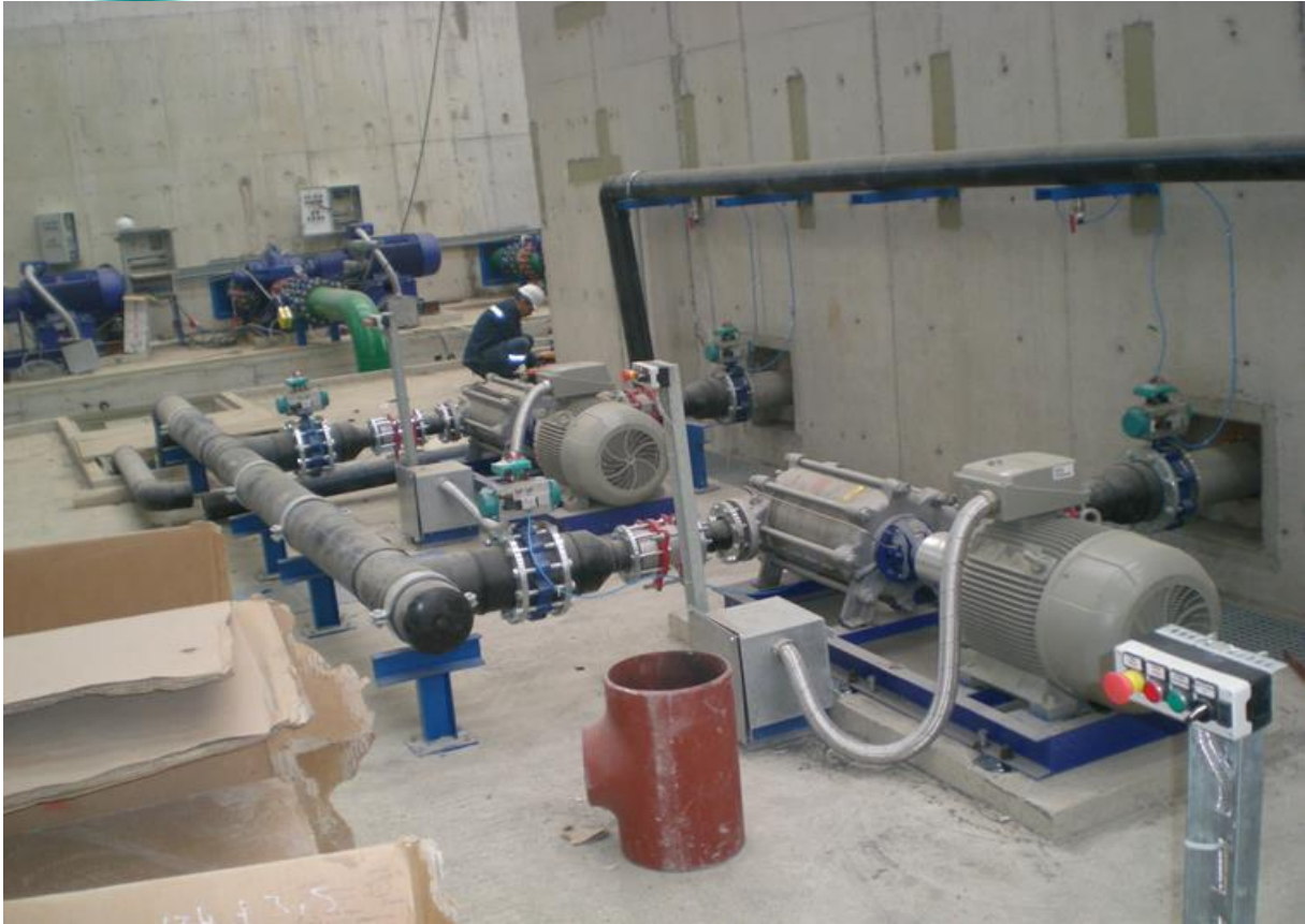
High Pressure Porcess Pump Installation
