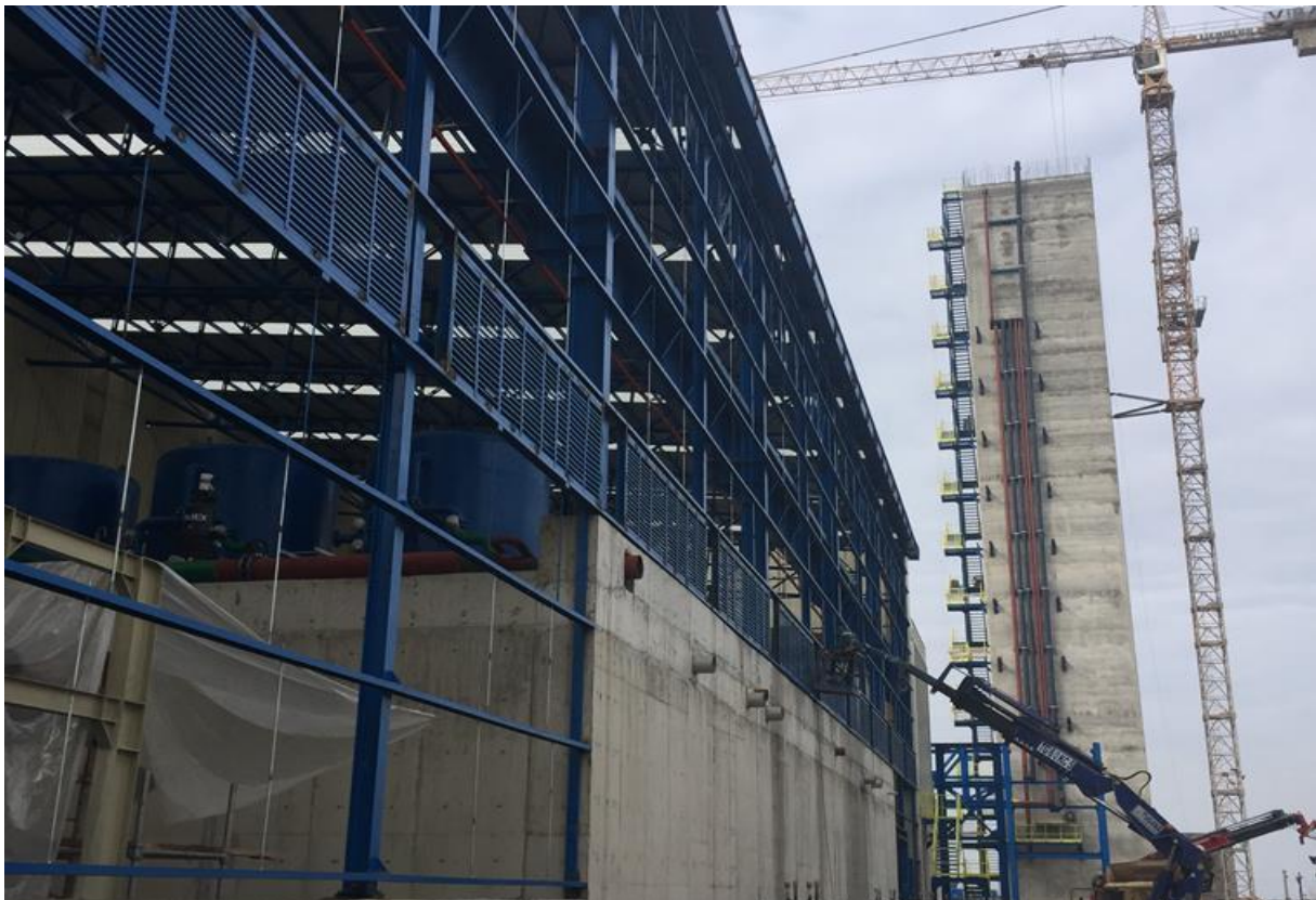
Water Treatment Area , Process and Emergency Water Basin Tower General Appearance
