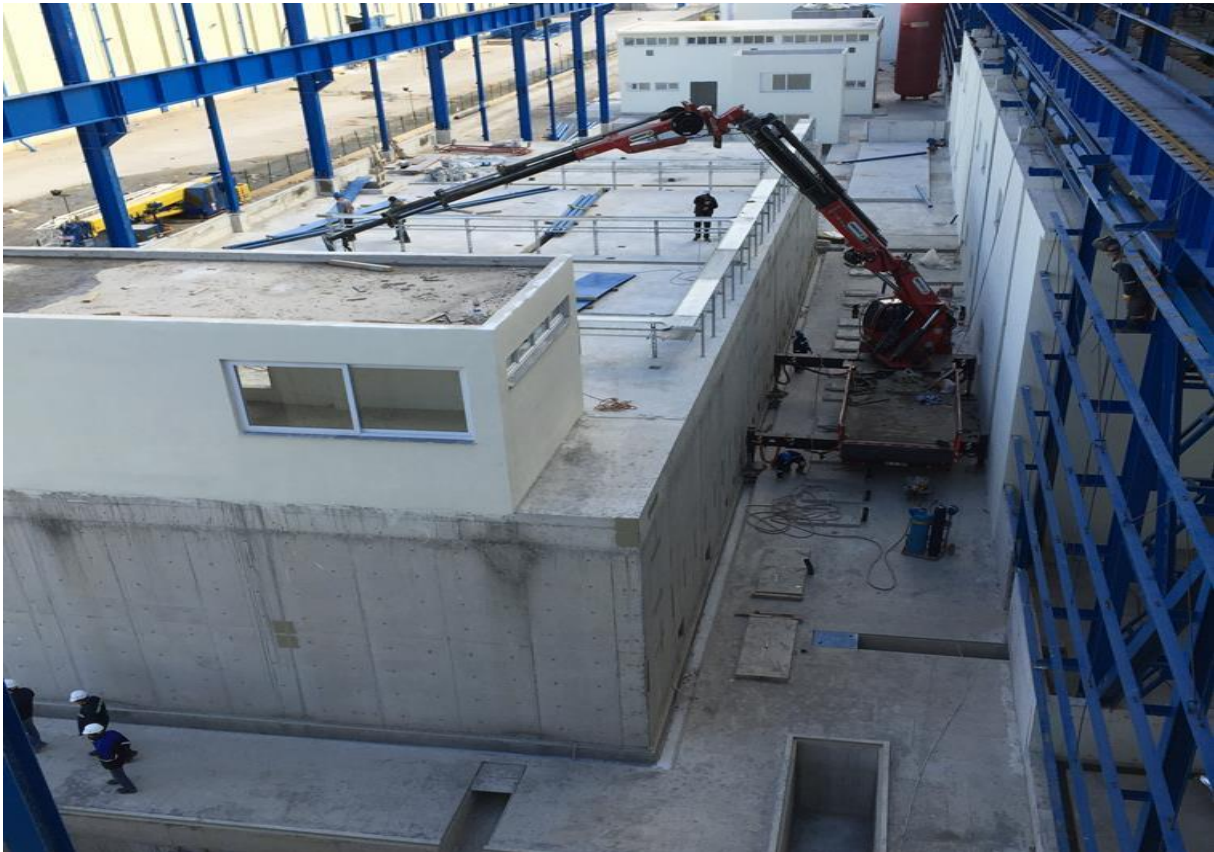
Process Water Treatment and Compressed Air Plant Area
