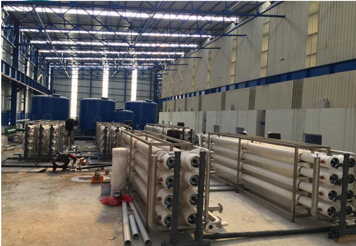
Sand Filters and Reverse Osmosis Area General Appearance
