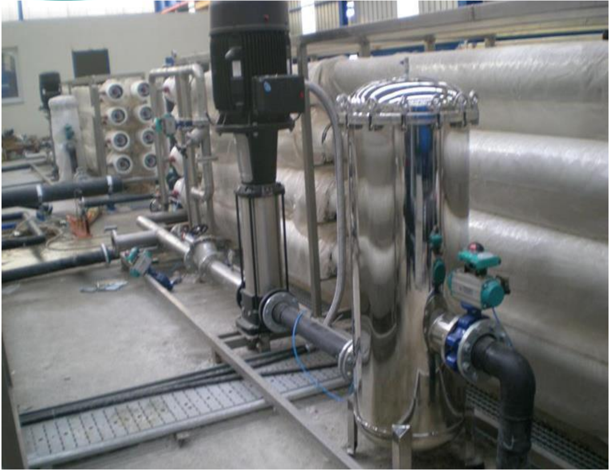
Reverse Osmosis High Pressure Pumps and Security Filter Installation
