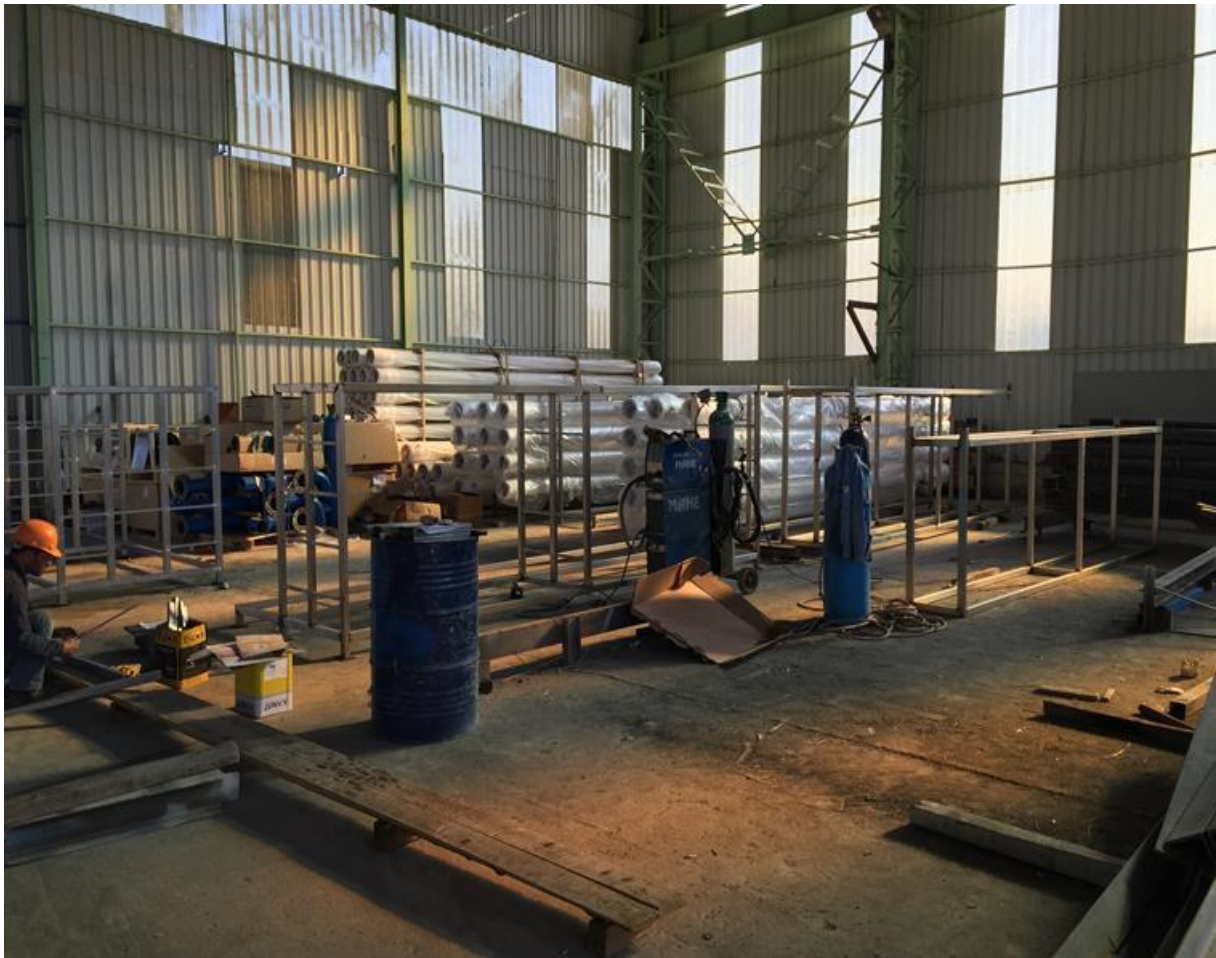
Reverse Osmosis Installation
