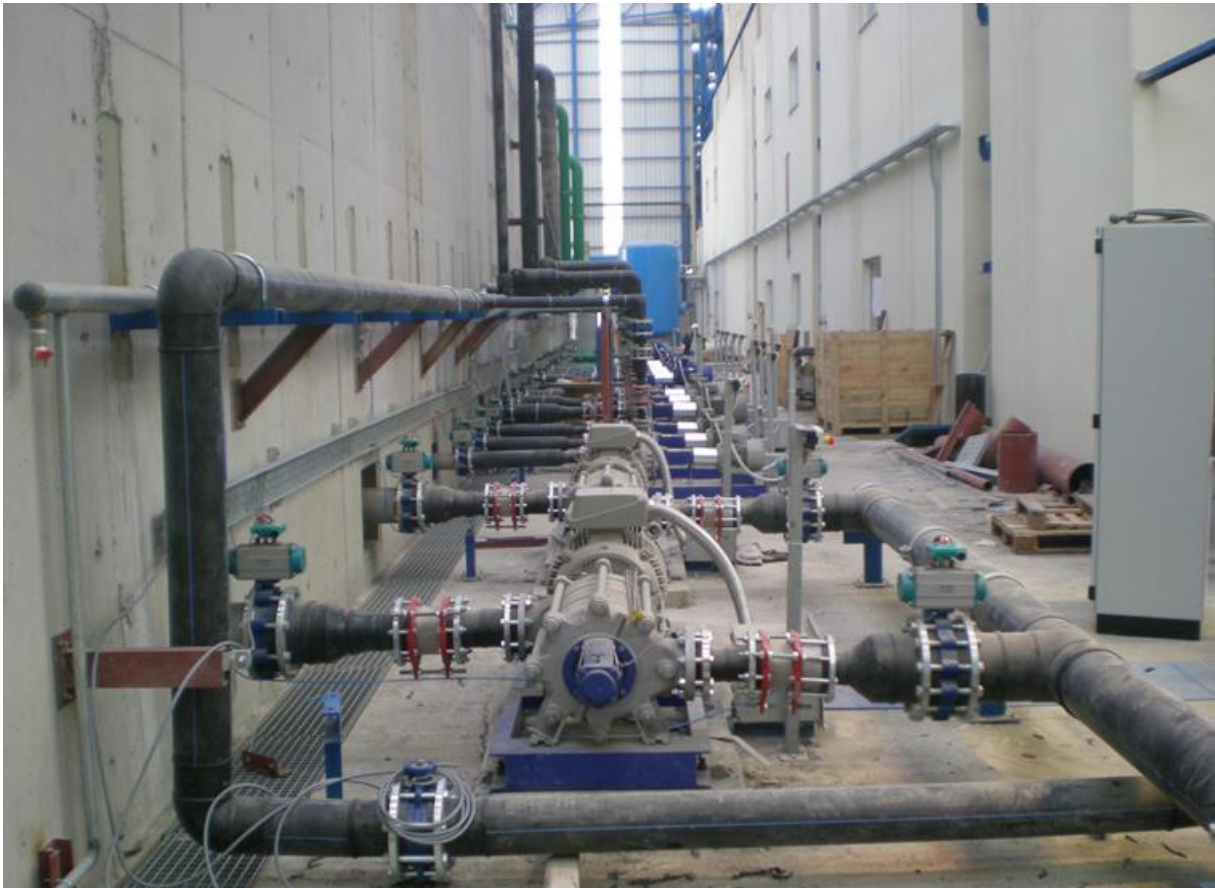
High Pressure Porcess Pump Installation
