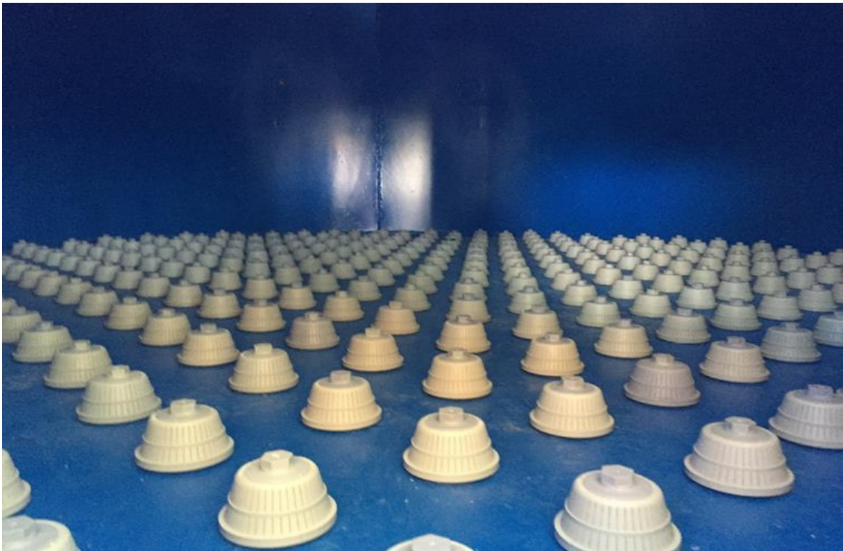
Sand Filters Nozzles
