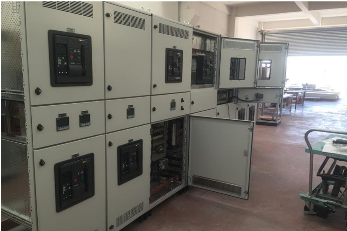
MCC /PLC Panel Installation
