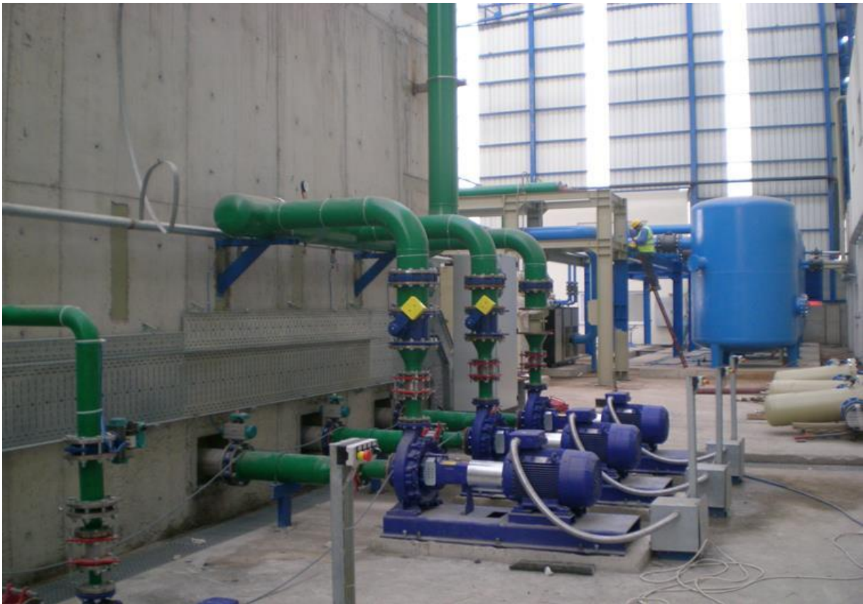
Compressed Air Plant and Sand Filter Pupms General Appearance
