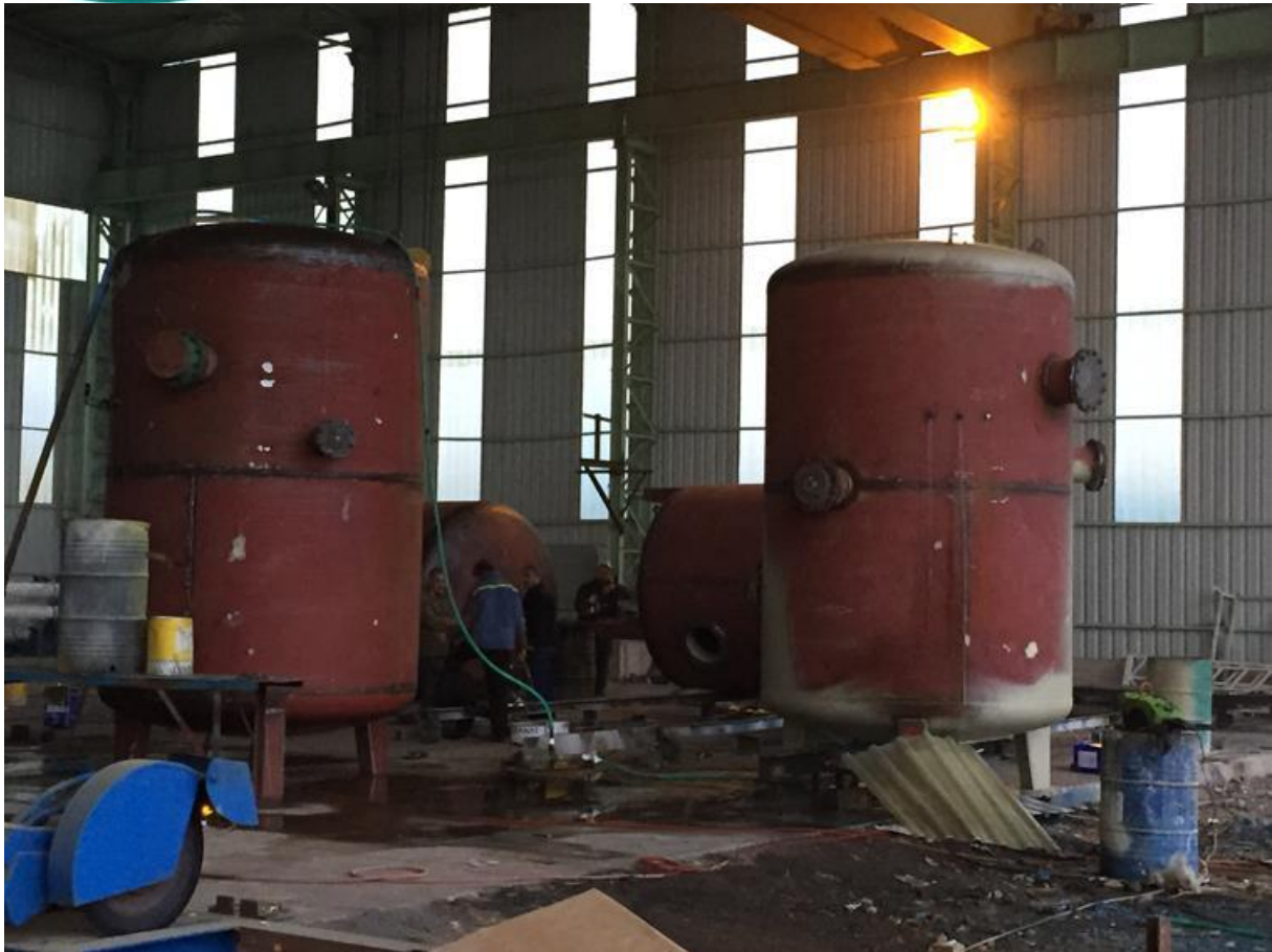
Compressed Air Plant Air Tanks Installation
