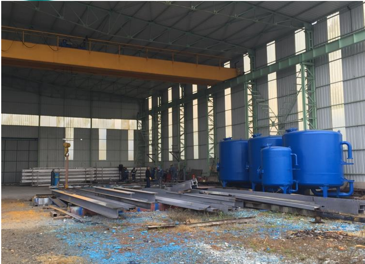
Reverse Osmosis and Sand Filter Installation
