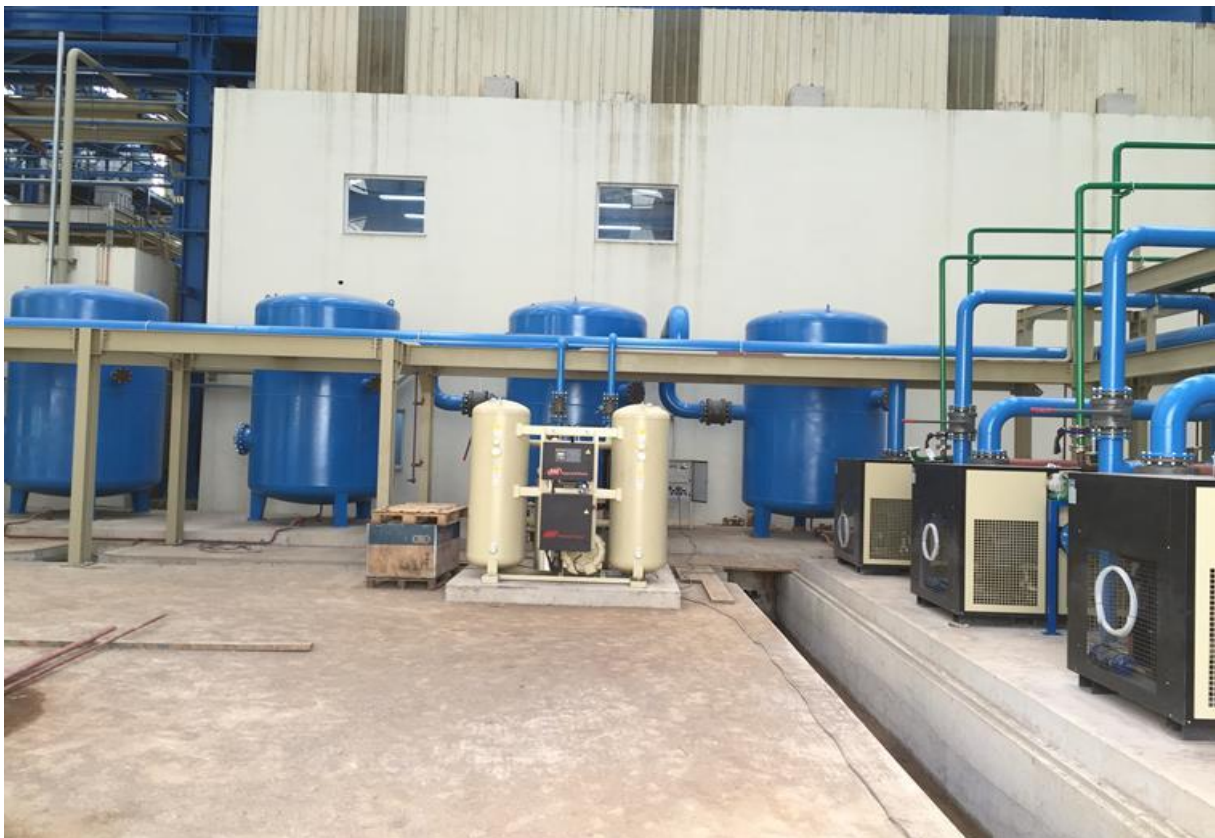
Compressed Air Plant General Appearance
