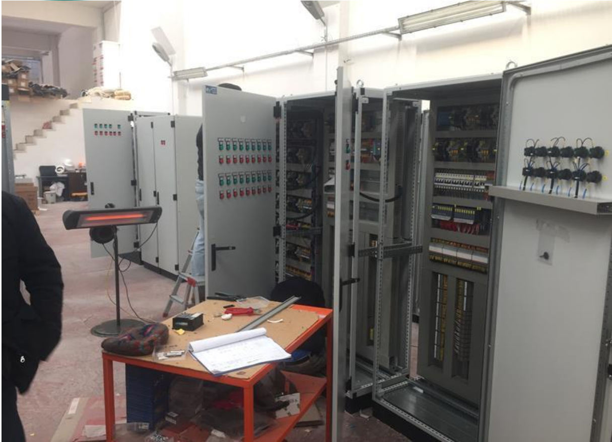
MCC /PLC Panel Installation
