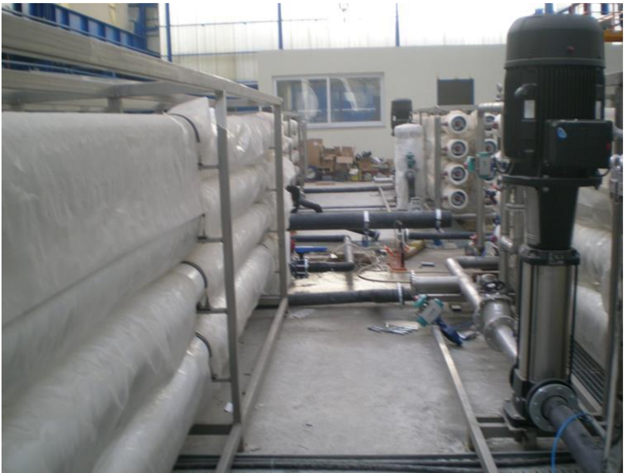
Reverse Osmosis Installation
