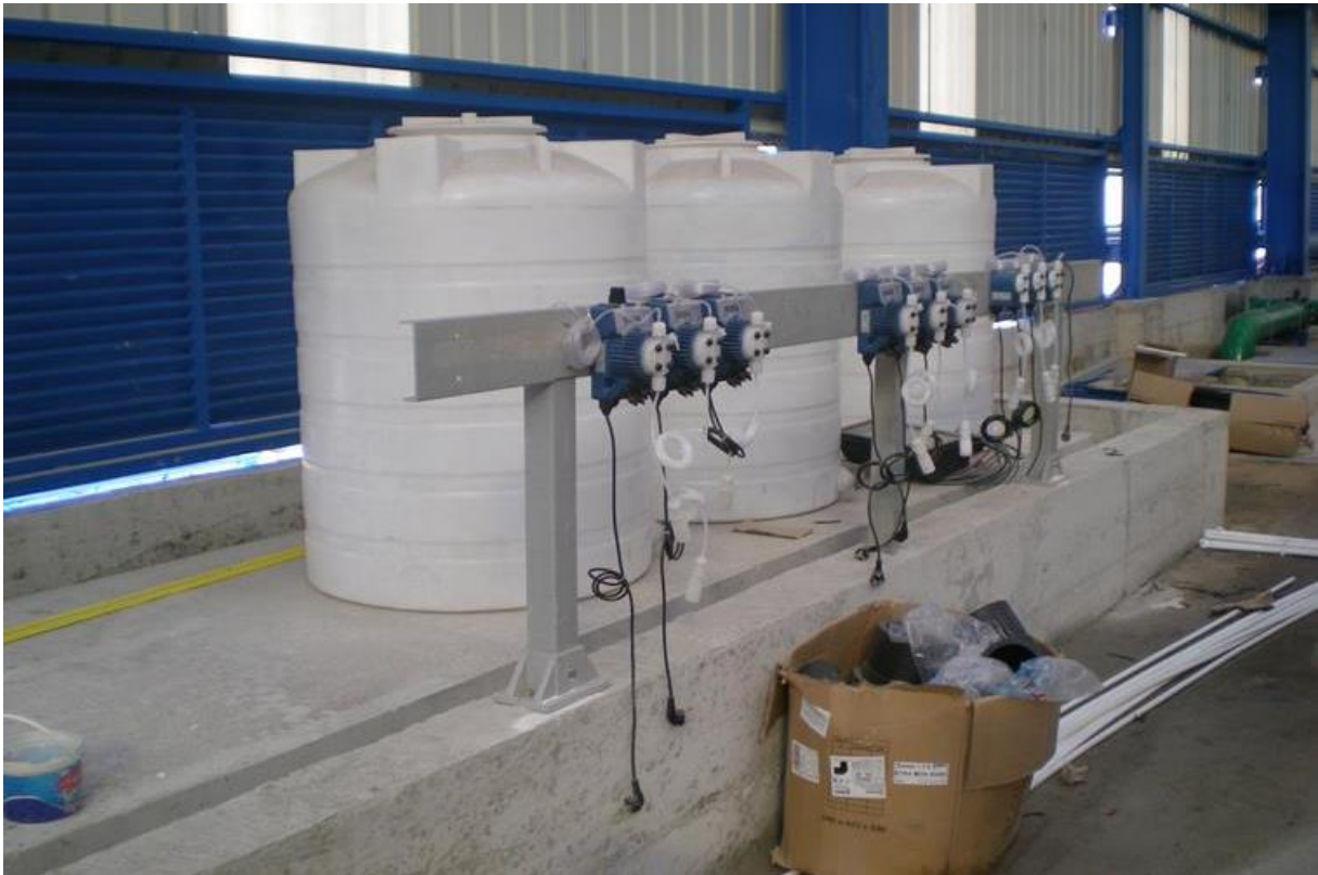
Chemical Dosing Unit Installation
