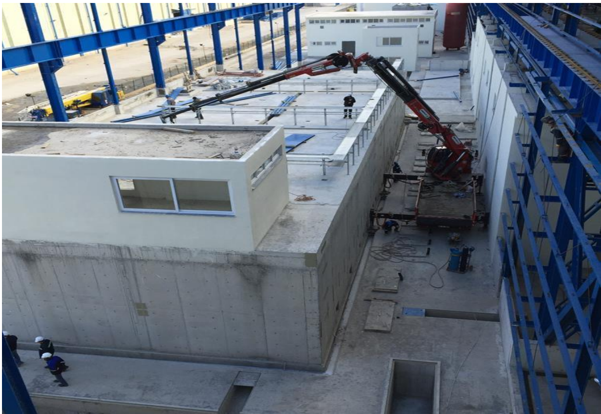
Compressed Air Plant (Upside) and Water Treatment Plant (Downside) General Appearance
