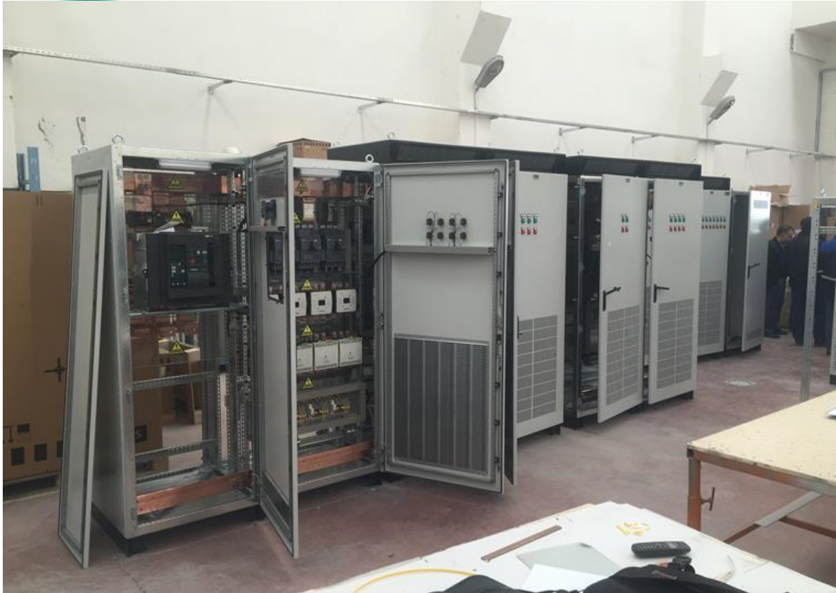
MCC /PLC Panel Installation
