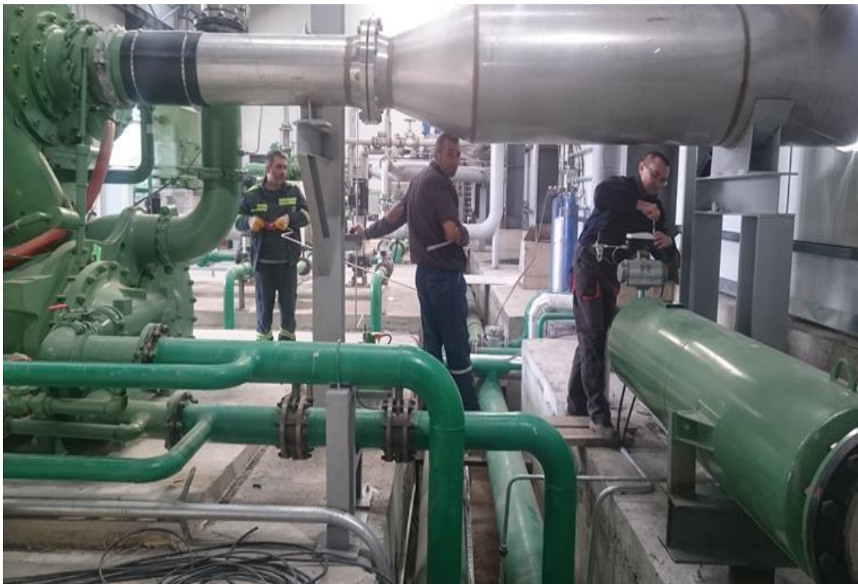
Main Compressor and Booster Compressor Commissioning with Supervisor
