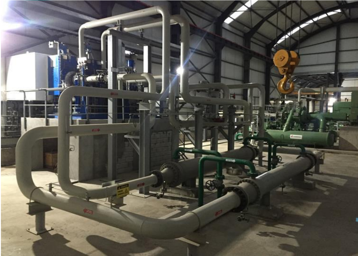
Main Türbine Commissioning with Supervisor
