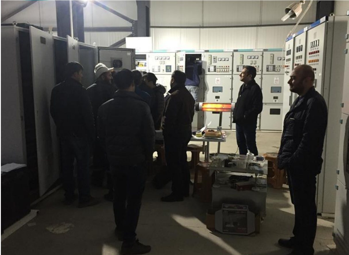
Electric Automation Commissioning
