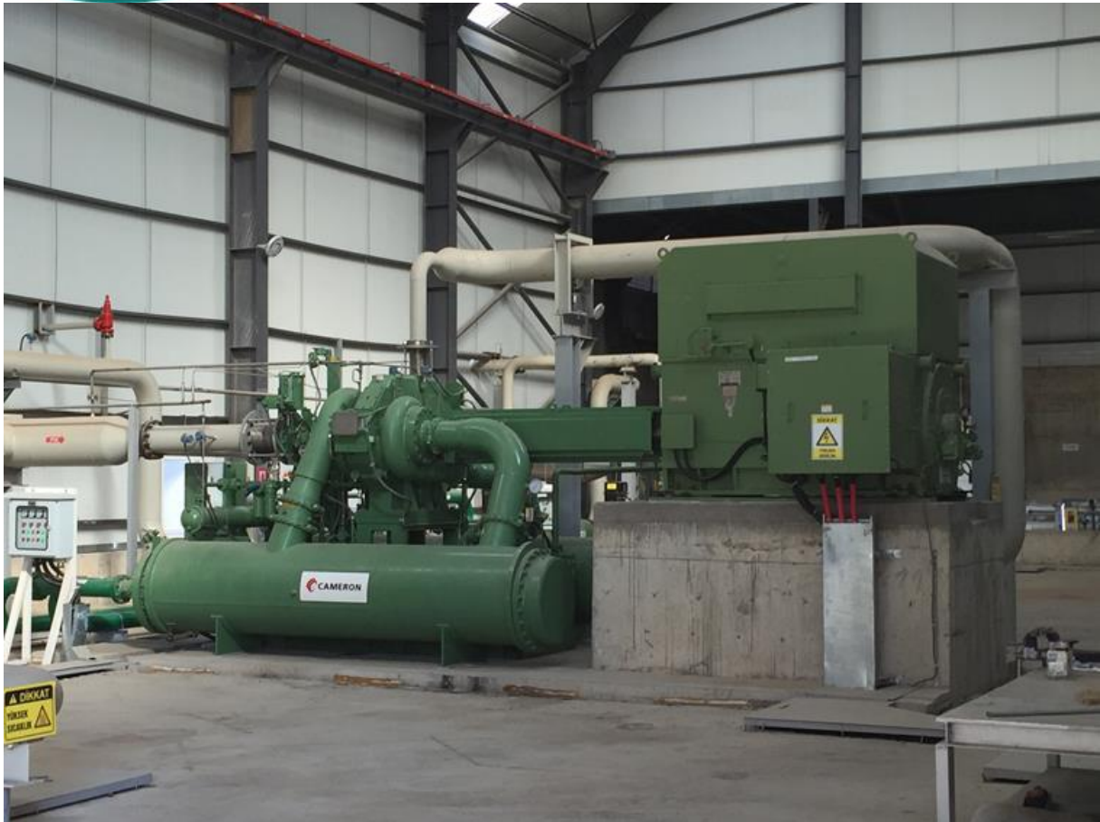
Main Compressor and Booster Compressor Commissioning with Supervisor
